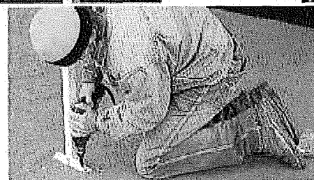
8. Secure base plates (that are attached to poles) to deck or concrete...
